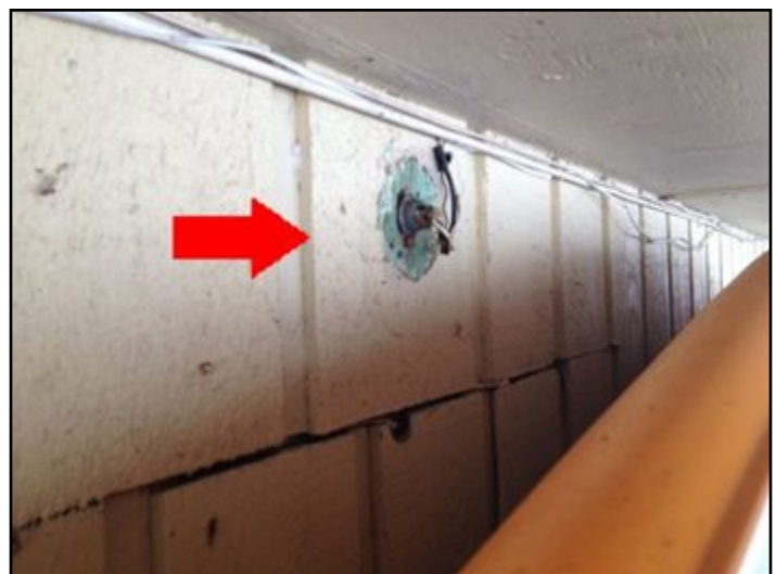
Live wires noted
