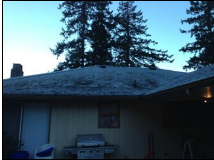
Moss noted on some areas of roof
