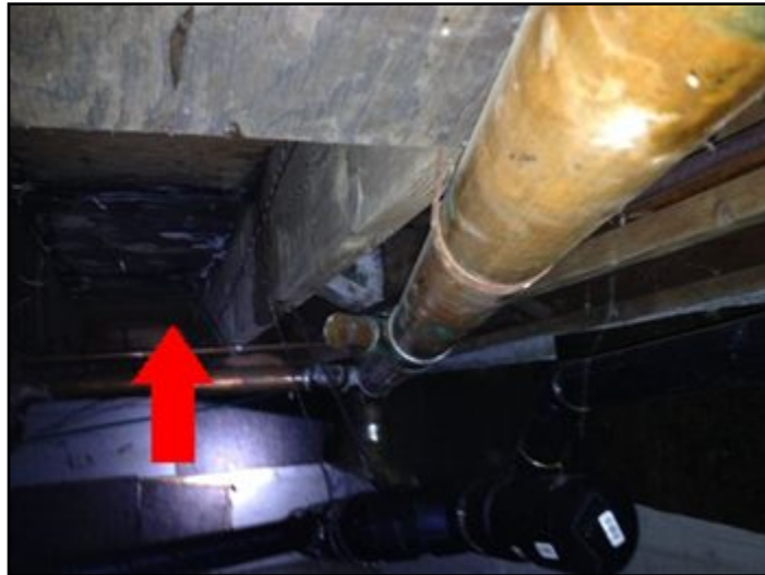
Water damage and rot noted
