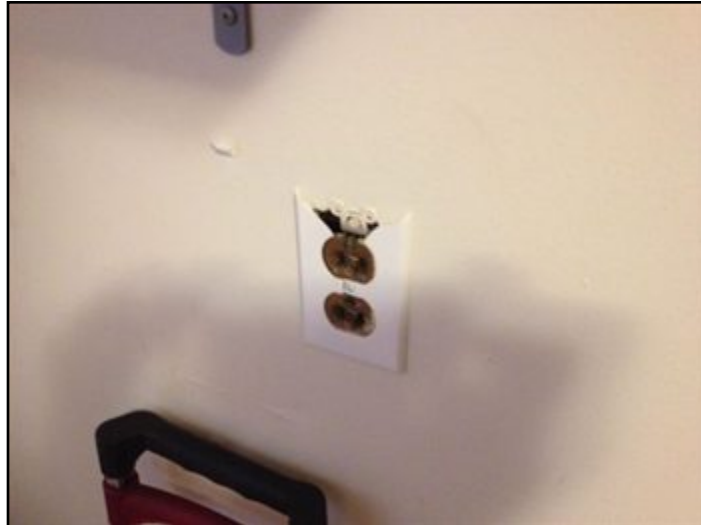
Damaged cover plate noted
