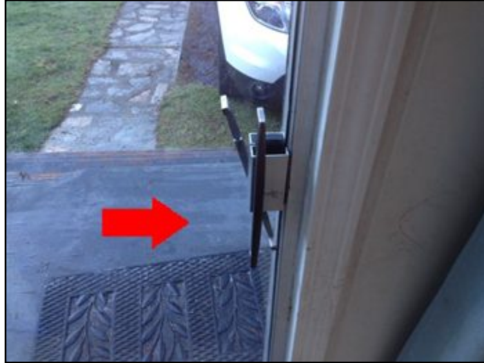
Door hardware damaged
