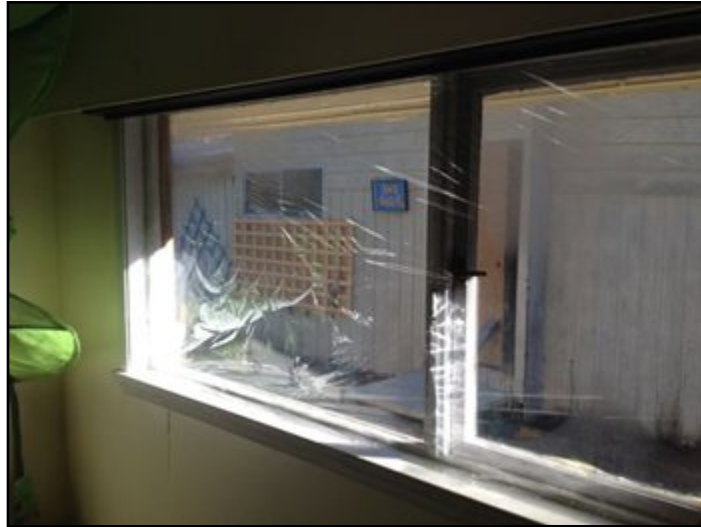
Plastic covering windows
