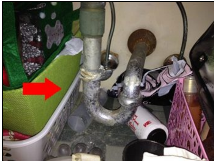
Rusty trap noted
