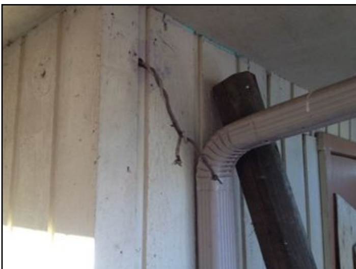
Live wires noted
