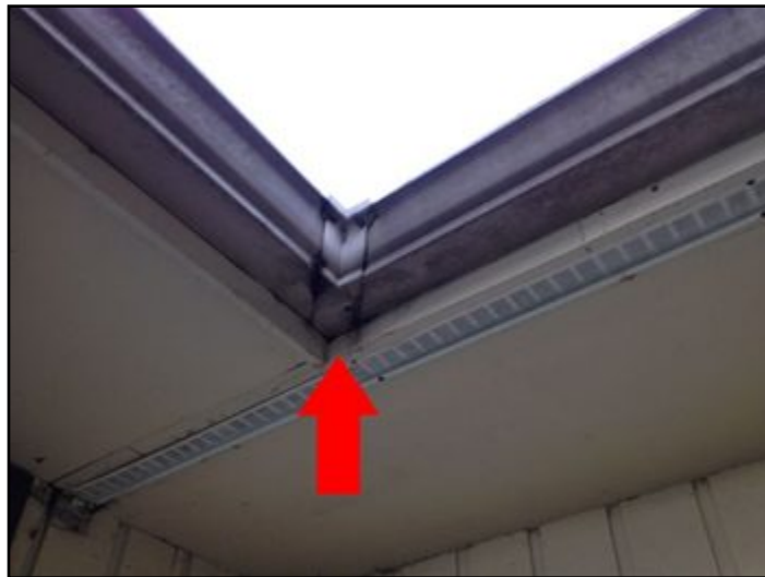
Various leaks noted
