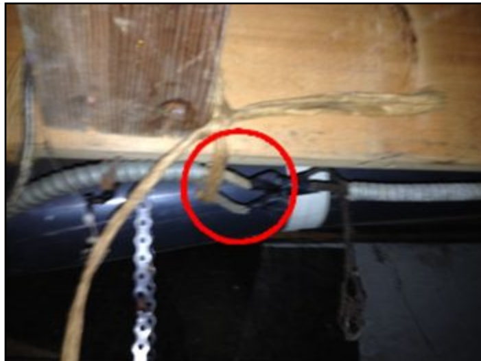
Exposed wiring connection
