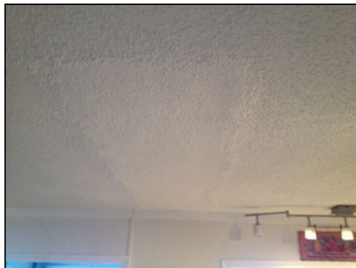
Ceiling patch noted
