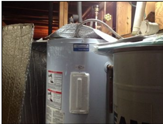
Hot water tank
