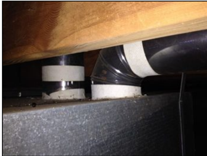
Tape may contain asbestos
