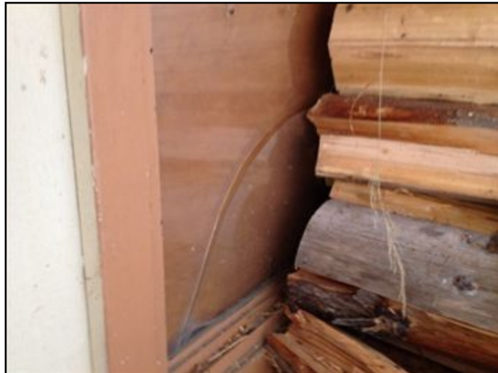
Broken window noted
