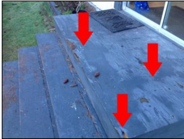
Rot noted. No weather protection.
