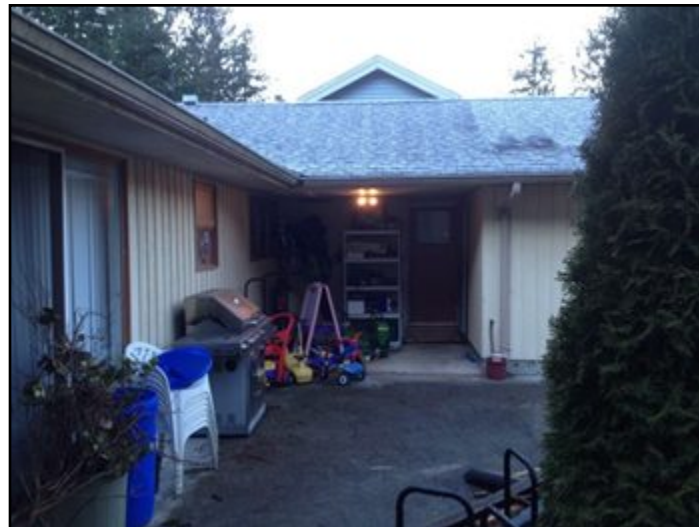
Ice on roof at time of inspection
