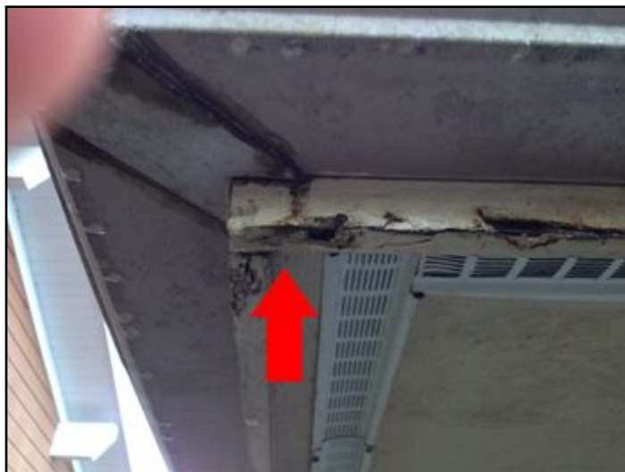
Face board rot noted
