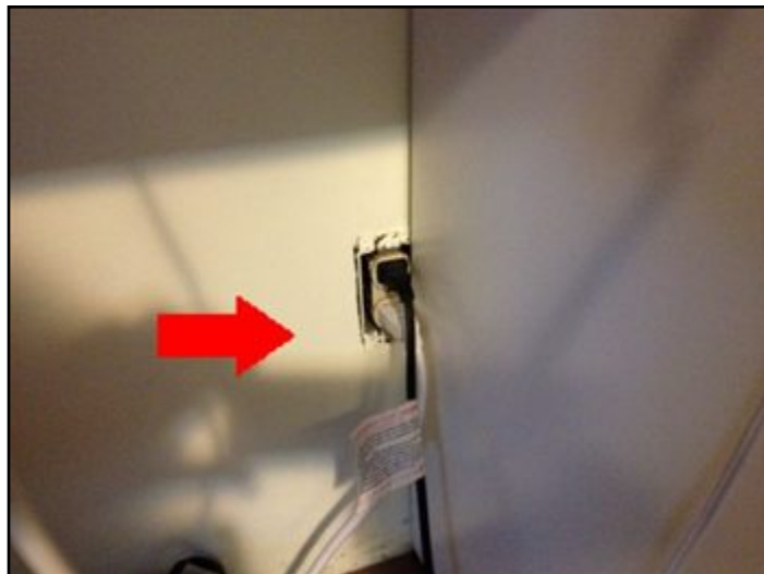
No cover plate noted
